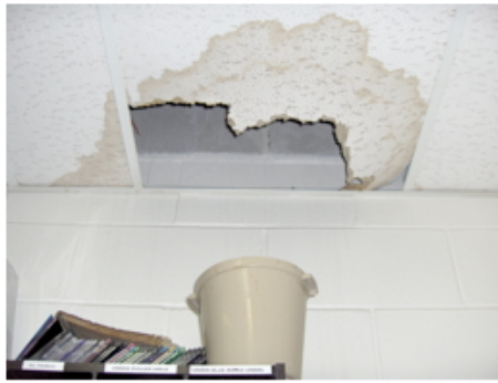
ANOTHER NEW HOLE IN THE CEILING
