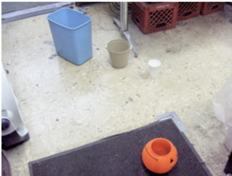
MORE BUCKETS FOR MORE LEAKS
