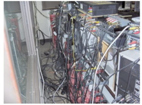
JUST WAITING FOR AN ELECTRICAL FIRE
